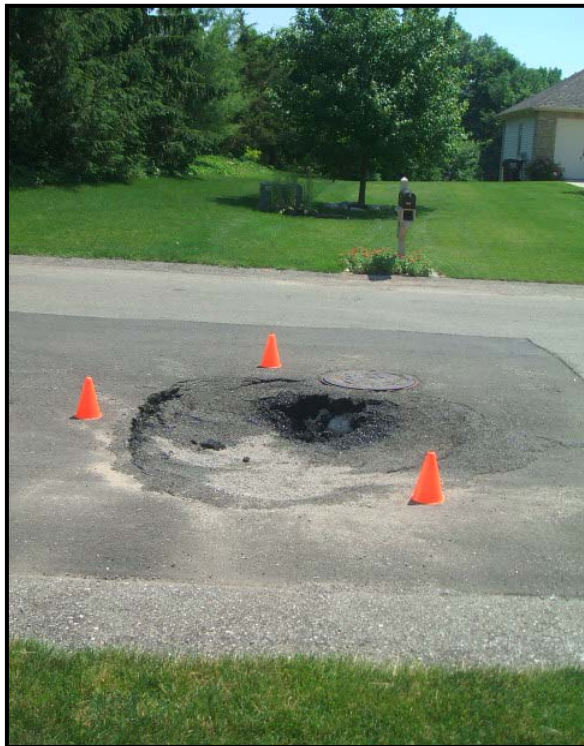
June 2009 Storm Damage
