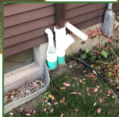
Sump pumps and roof drainage with no positive outlet point
