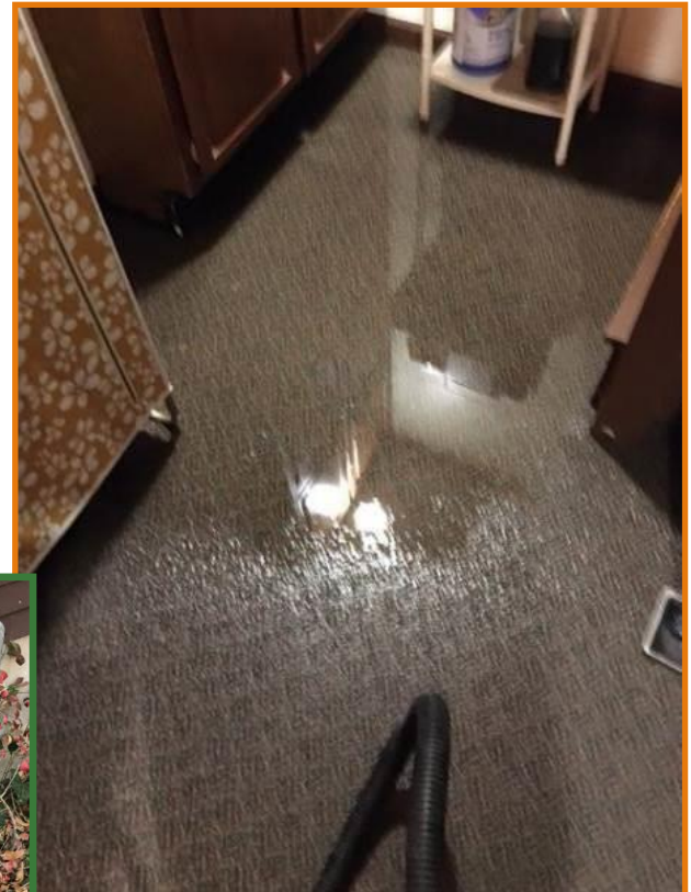
Flooded basement of 16215 Terrace Road
