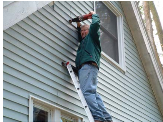
Photo: Dale Congdon helps to weatherize a home. Here he is drilling a hole to install a vent.
