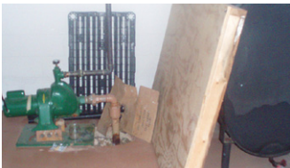
drinking well next to a fuel oil tank
