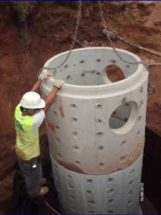
Infiltration Catch Basin
