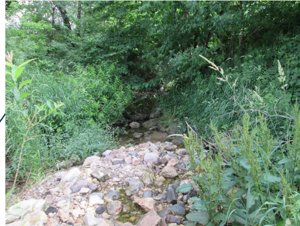
Looking downstream (north) at riprap fallen into the drain channel
