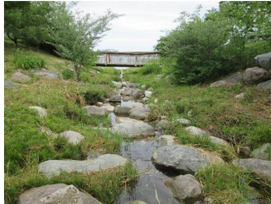
Looking north toward the lake from the Van Buren Street box culvert outlet
