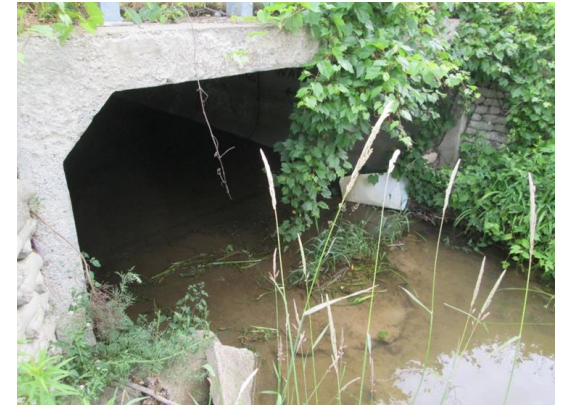
Looking northeast at the inlet to the Van Buren Street 7' x 16' box culvert
