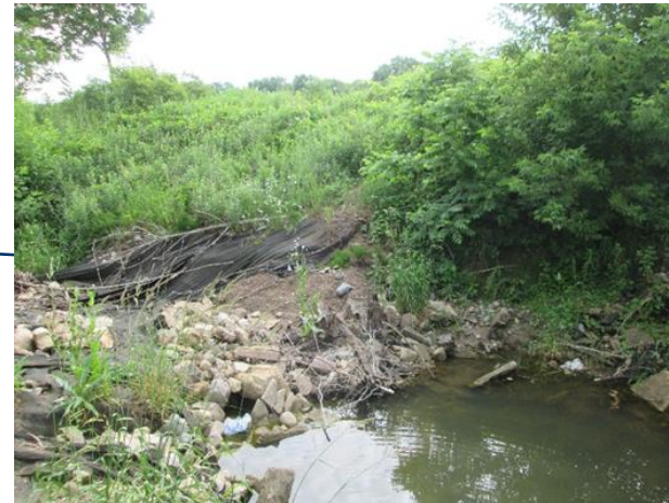
Looking east from the Barry St. culvert outlet with a scour pool shown in the bottom right of photo
