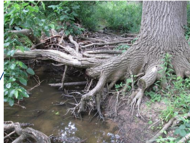
Looking upstream at the Barry Street 6' x 12.5' box culvert with a large scour pool at the bottom of the photo
