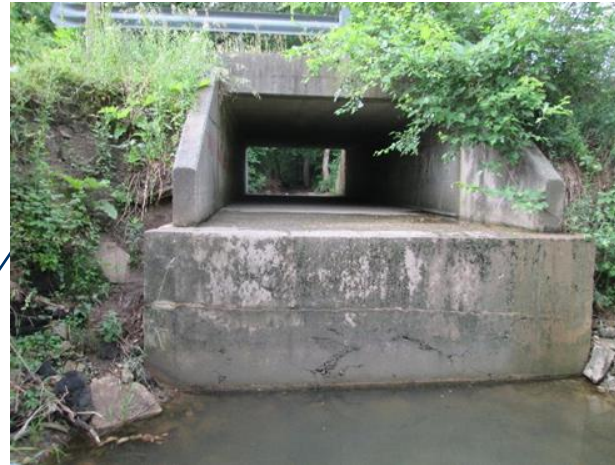
Looking upstream at the Barry Street 6' x 12.5' box culvert with a large scour pool at the bottom of the photo
