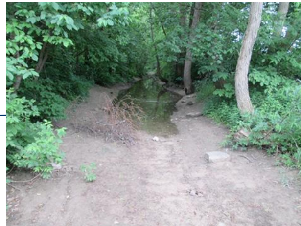
Looking upstream from the inlet to the Barry Street box culvert demonstrating the improperly graded channel south of Barry Street
