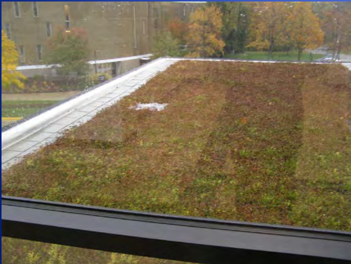
Green Roof on Mackinac Hall
